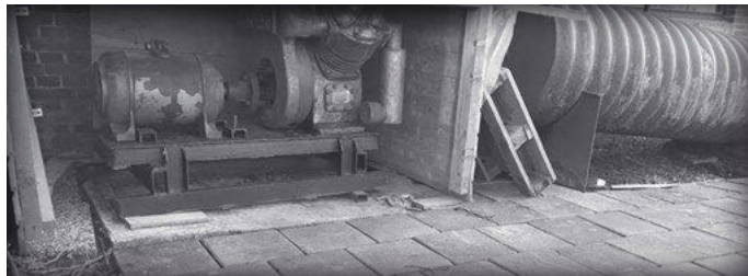
Compressorhok met expansievat
